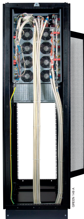
Rear view (before adding rear protective cover). Flexible cabling management for easy connections and tidier cabling.
