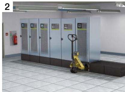
600 kW, mode on-line double conversion
